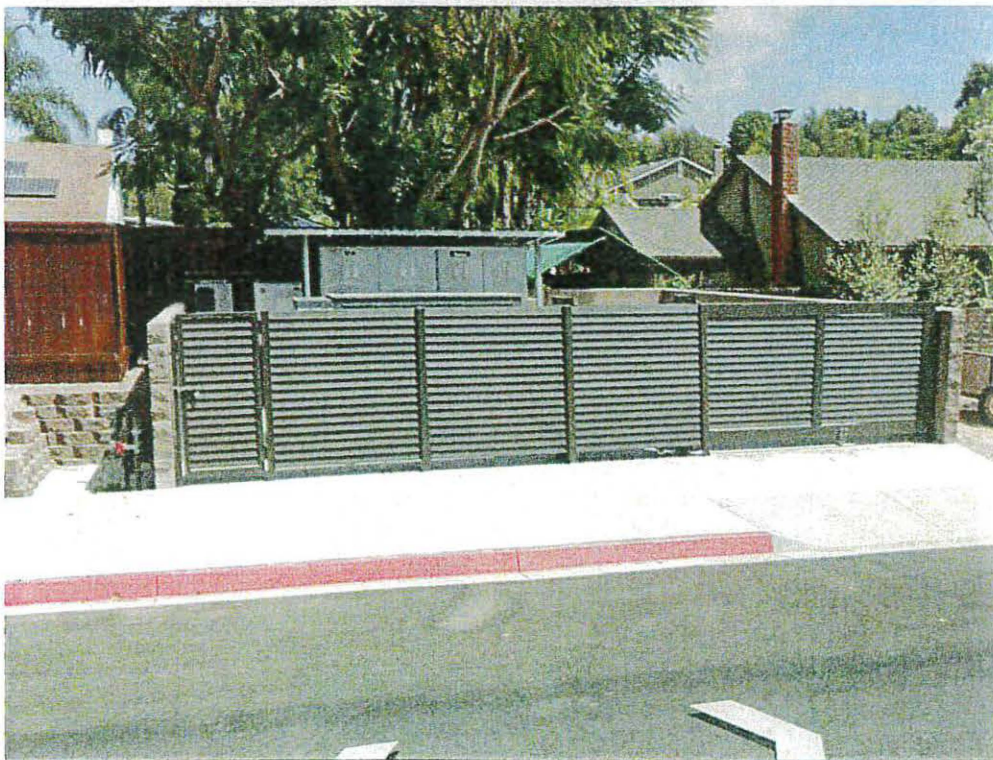
Fig 4. Example screened pump station site (LWD Encinitas Estates)
